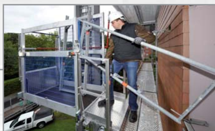
Stor lasteplatform (1,40 x 0,85m)
